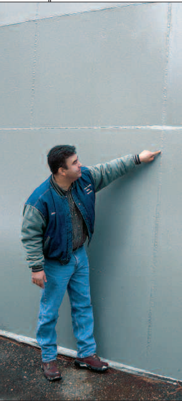
Getting an up-close look at a tank seam is James Alarid, an engineer with the Los Alamos County Department of Public Utilities. The seam is the result of an opening painters had cut into the tank wall to move equipment and personnel inside (right).
