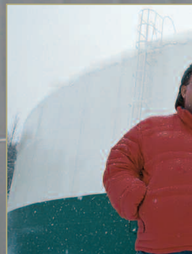
A painter applies Fast Clad Zinc HS to cleaned and blasted steel on the surface of a 5-million-gallon water tank in Anchorage, Alaska. Above, AWWU engineer Sid Taylor and the finished tank brave a snow shower.
