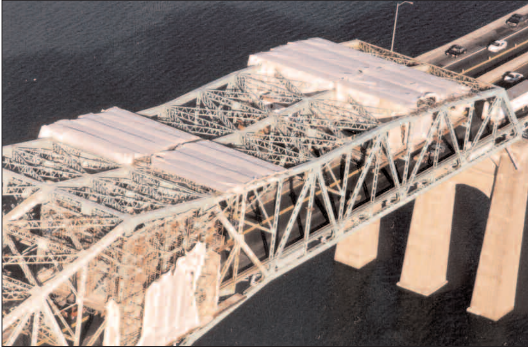
Visible above is a work in motion. The scaffolding at left has been moved into a new position, and the "rolling roof" will soon follow. The enclosed area at right contains painters at work at the time of this photograph.
