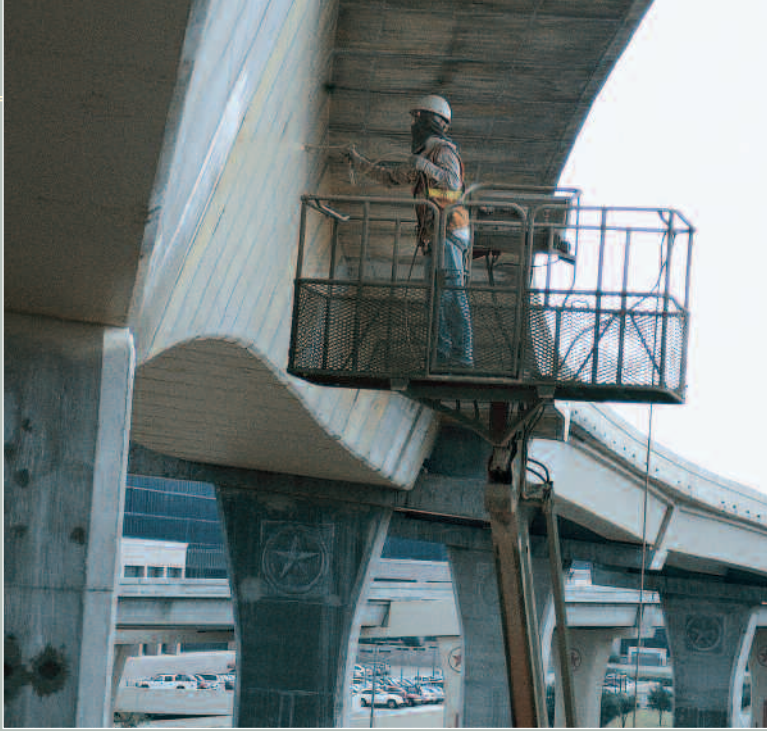
Manlifts were used to raise painters to the top levels of the interchange, which reached heights of 100 feet.
