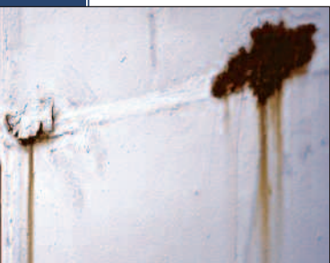
Above (top), water collected in a variety of areas aboard the Yorktown, leading to corrosion. Rust streaking was also a common occurrence on vertical surfaces.
