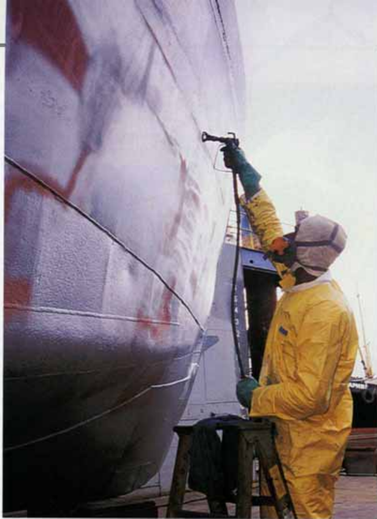
The Icy Bay (above and lower right) receives a coatings system designed to withstand the rigors facing a commercial crab boat.
